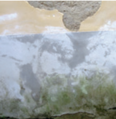
Wall with saline efflorescence to be restored with Albusil Antisale
