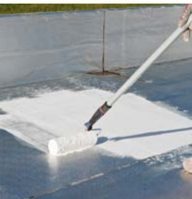
Application by roll or brush of one or more coats of Guaina Liquida Fibrata of Plastimur.
